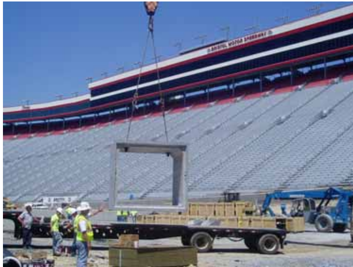
A section of 9' x 8' precast concrete box culvert being unloaded at the project site at Bristol Motor Speedway.
