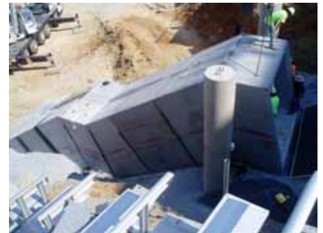
Precast box culvert being installed as a pedestrian tunnel with grade changes and varying fill heights.
