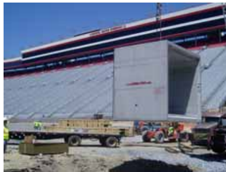
A section of precast concrete box culvert at the Bristol Motor Speedway job site.
